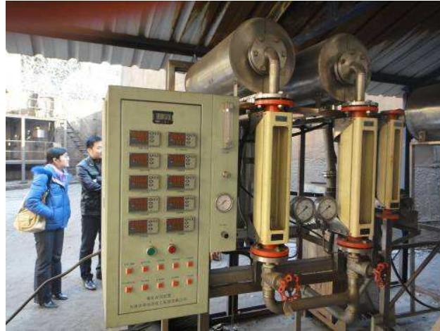
Visiting SCR-Dioxin Reduction Testing Facilities in iron sintering plant, Jinan, Jan 24, 2011
